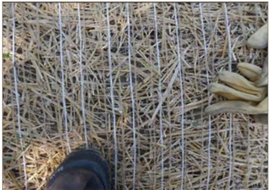
Erosion Control Fabric with a Biodegradable Mesh
