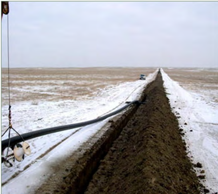
Minimal Disturbance Pipeline Constructed During Frozen Ground Conditions With No Soil Stripping
